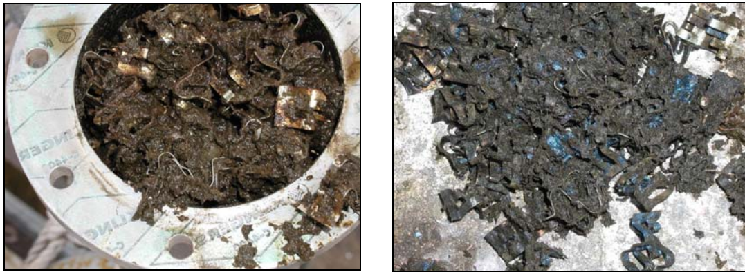
Figure 10 Steam stripping – clogged column with solid material
