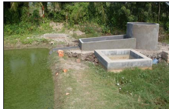
Figure 5 Leachate holding tank, bio-filter and leachate pond
