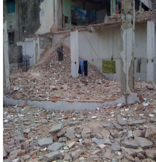
Figure 4 Rubbish & concrete pieces
