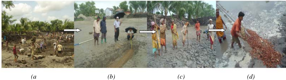
Figure 6 Construction of base liner. Execution of (a) earth excavation, (b) leachate detection system, (c) preparation of CCL and (d) placing of leachate collection pipe
