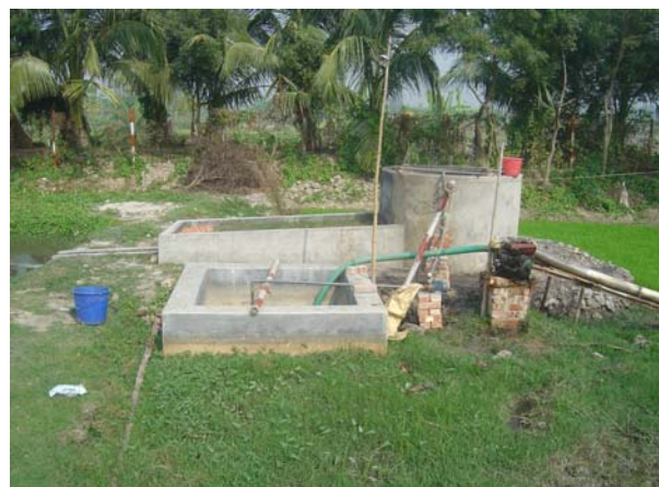
Figure 11 Leachate holding tank which collects leachate from the cell through gravity flow
