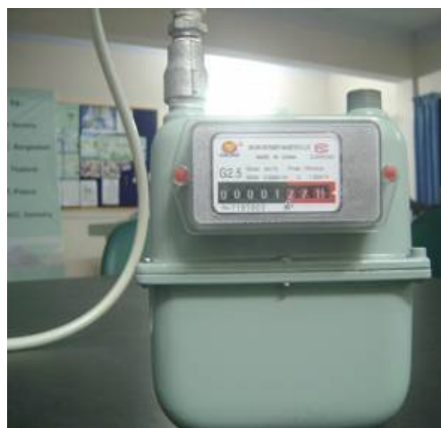
Figure 13 Flow meter device
